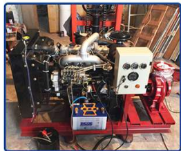
DIESEL FIRE PUMP
