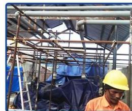
INSTALASI PIPA HYDRANT
